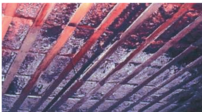
Ceiling of a refrigerator warehouse contaminated due to the accumulation of dust and condensation.
