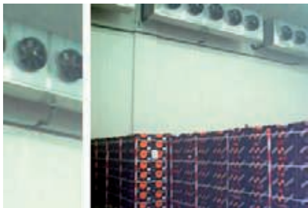
Pre-cooling in a pre-cooling tunnel of oranges and clementines, packaged in crates, labelled and placed on disinfected pallets, before being moved to the cold storage room where they will remain until being shipped.
